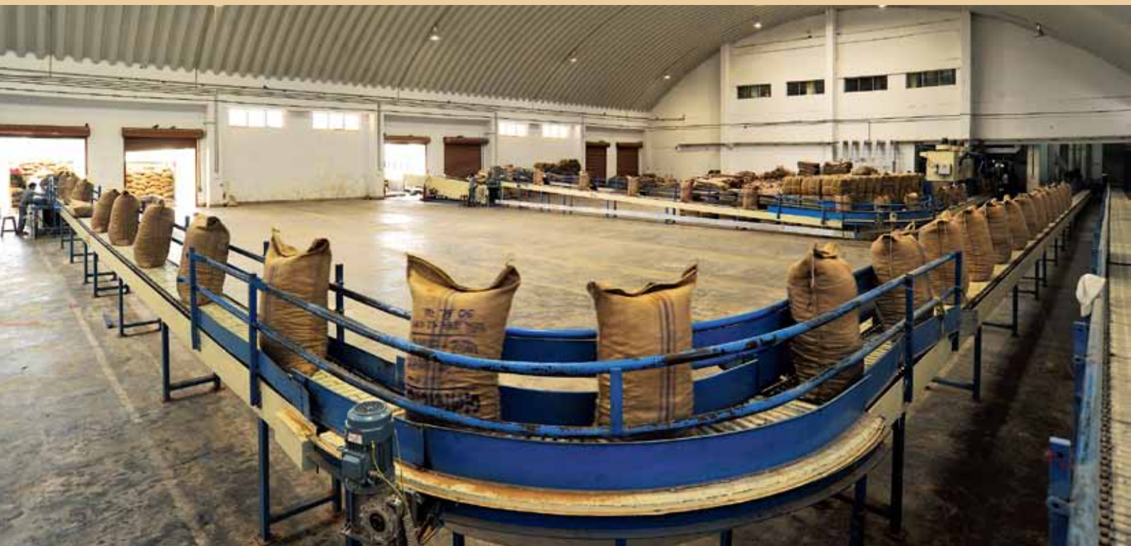
An automated packing and despatch line for the 1,000 MTPD cattle feed plant.
